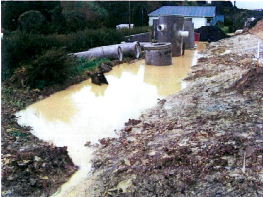
Figure 1 – Poor subdivision earth works management
