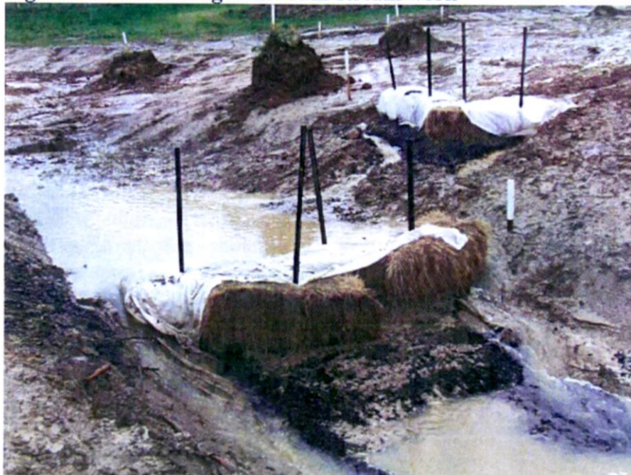
Figure 2 – Poor management of in-stream work
